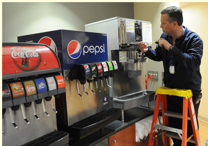
Luis Marrero, an air conditioning and refrigeration technician, works on an ice machine in the doctor's lounge.
